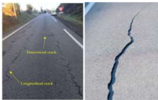
Fig1(Types of Road Damage)
